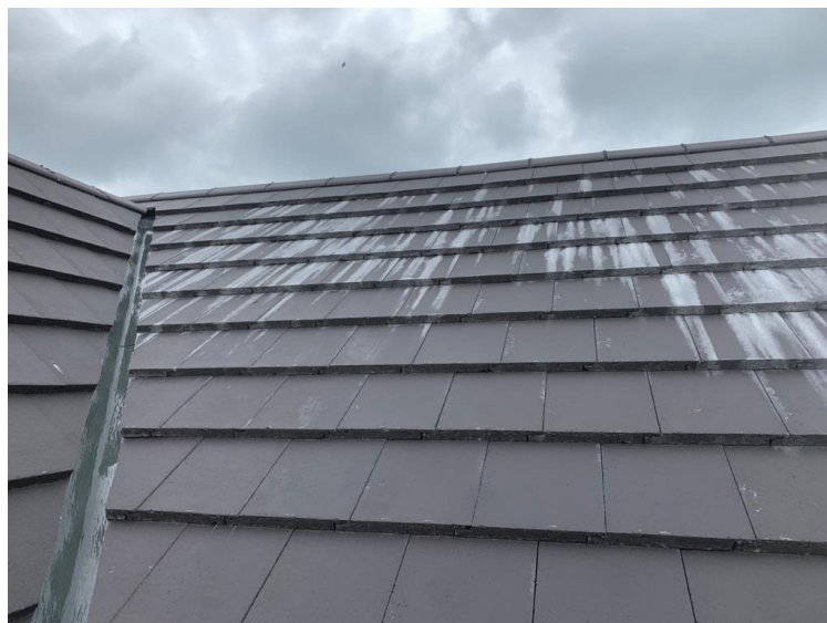
Figure 5. Example of concrete roof tiles exhibiting efflorescence streaking
