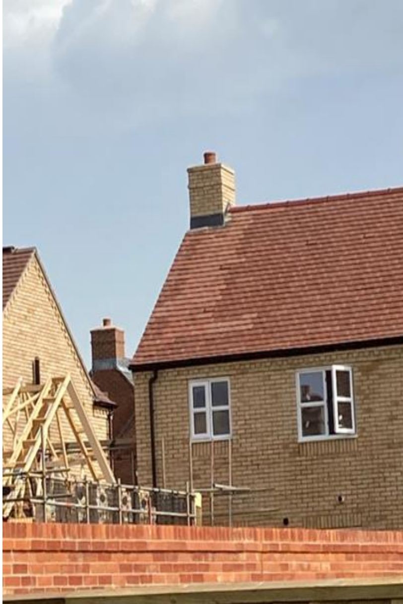
Figure 1. Example of poor concrete roof tile mixing
