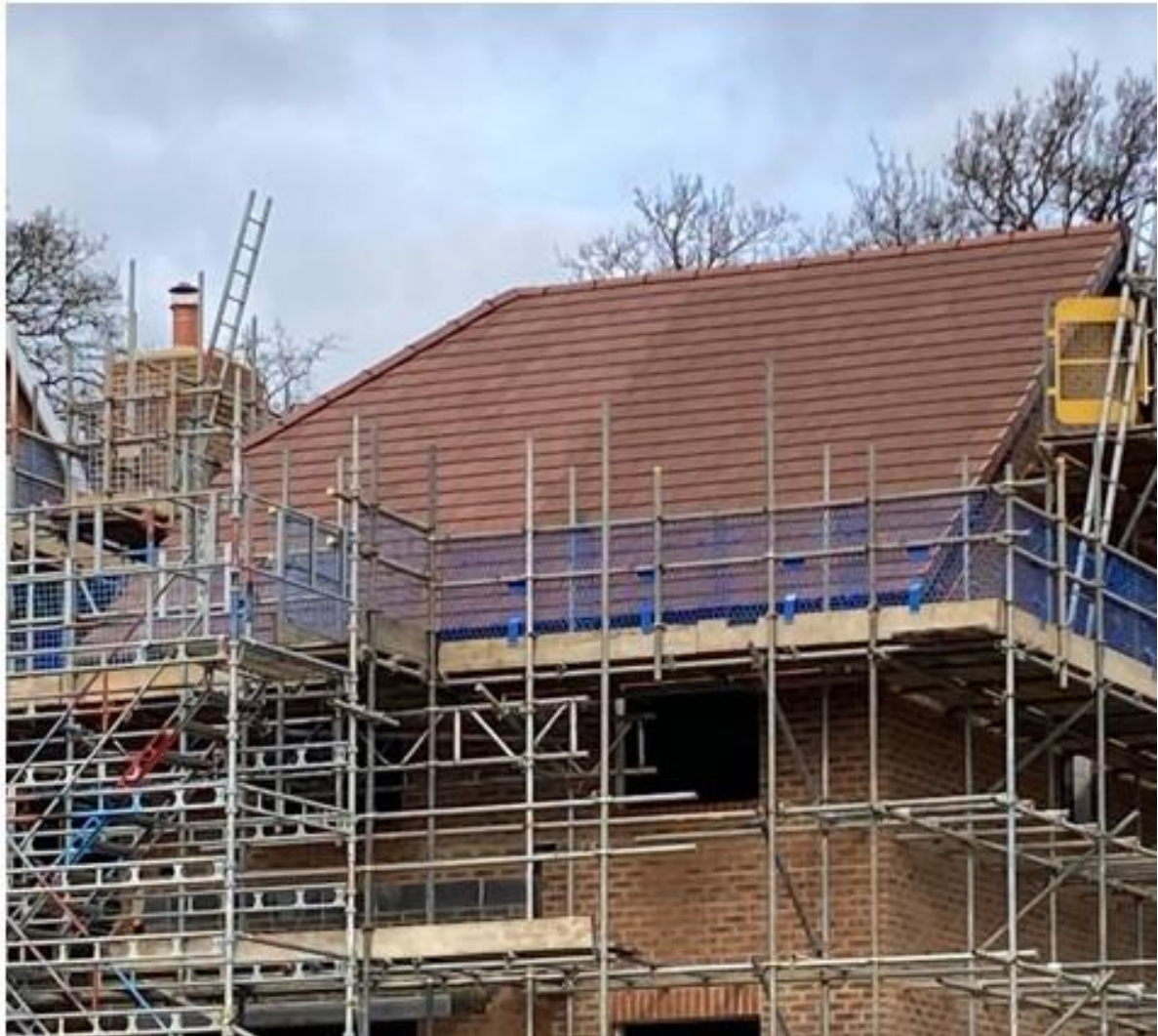
Figure 2. Example of poor clay roof tile mixing
