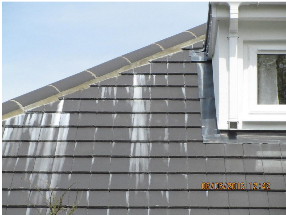
Figure 6. Example of mortar from hip tiles causing efflorescence
