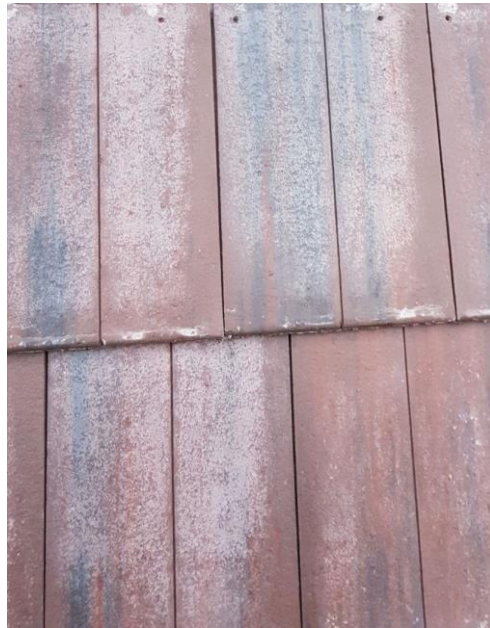
Figure 4. Example of concrete roof tiles exhibiting efflorescence bloom
